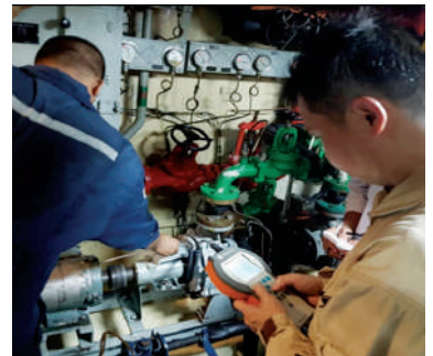
Figure 4. Vibration Data Acquisition On Board KD JERAI.
